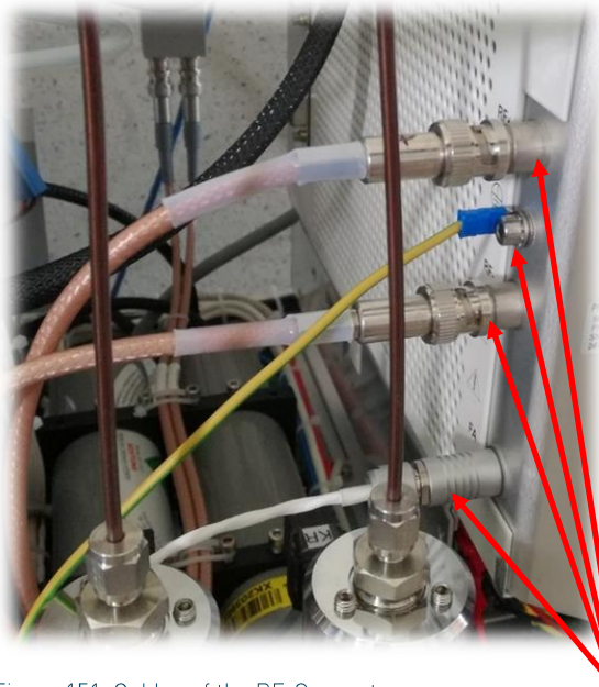
Figure 151: Cables of the RF-Generator
