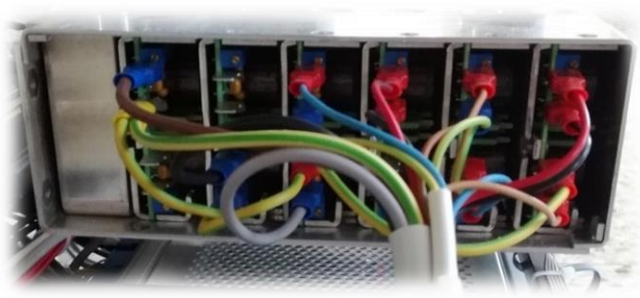
Figure 144: Outlets of the power supply
